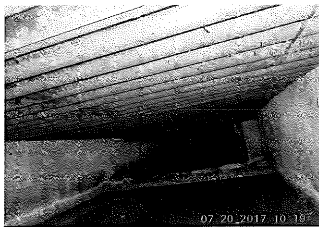
VIEW OF RETURN AIR SYSTEM AFFECTED WITH PONDING WATER
